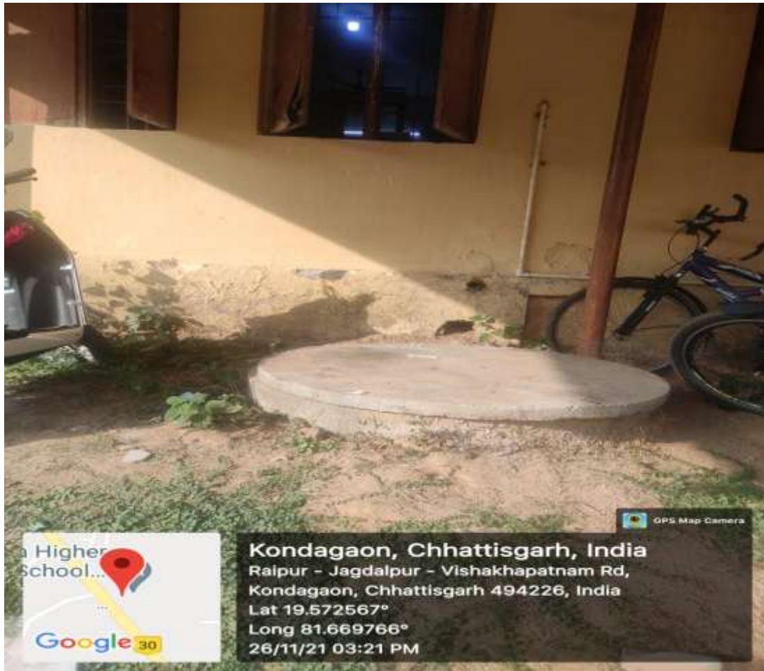
Fig.: Soak-Pit attached with chemistry lab
